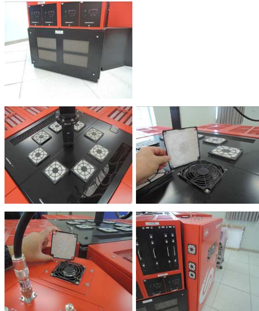
Cleaning of the air filters for SSPA Transmitter
