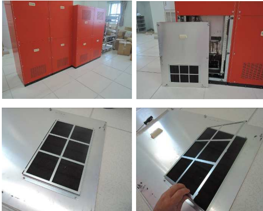
Cleaning of the air filters in the DRSP
